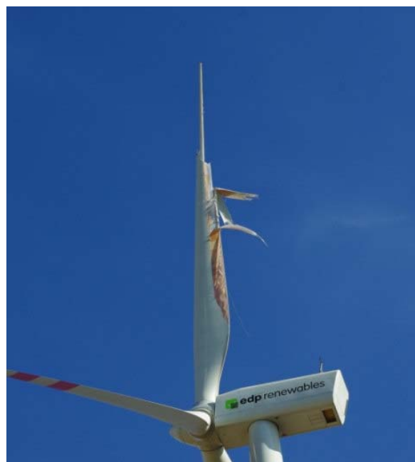
Damaged blade of a wind turbine (source: Gamesa technical report)
